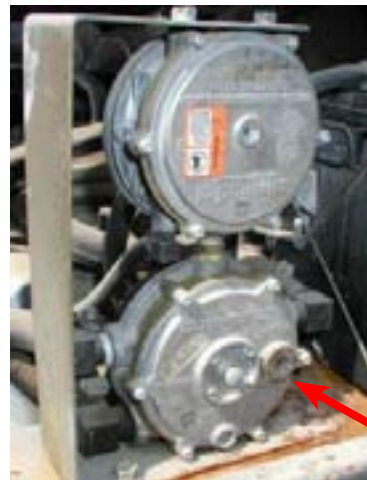
Figure 86. Drain plug and vacuum fuel filter lockoff on a simple vaporizer
