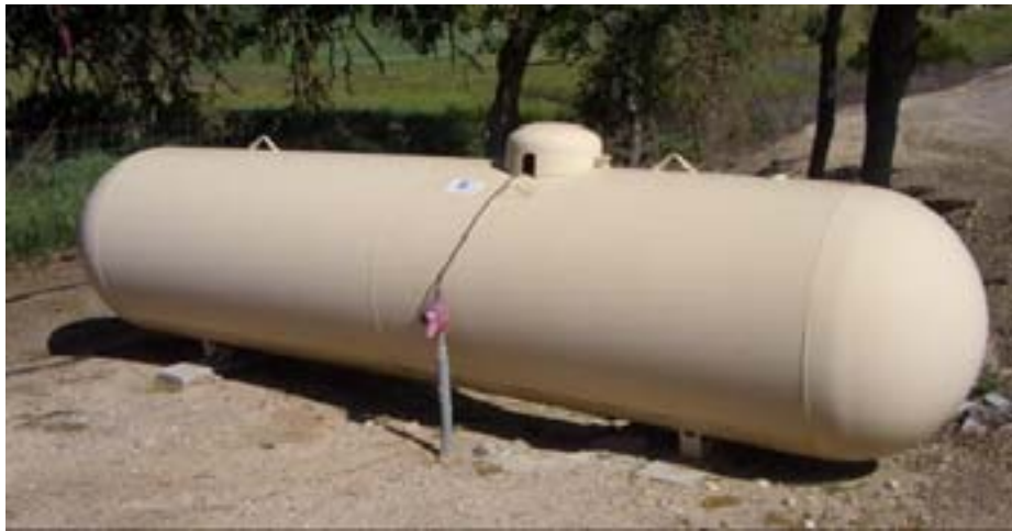
Figure 45. Vapor service tank with first-stage regulator
