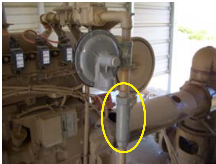
Figure 87. Cartridge filter in vapor supply line
