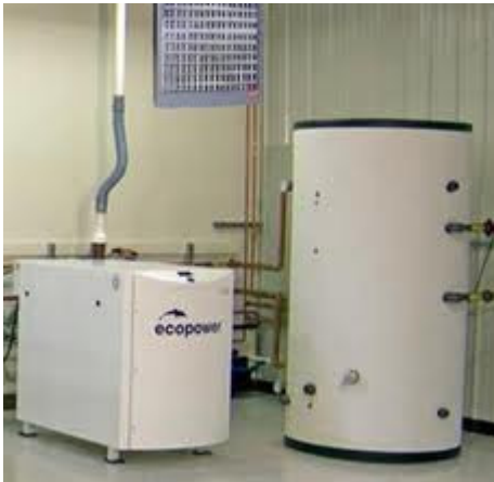
Figure 9. Marathon Ecopower residential CHP unit with a water buffer tank
