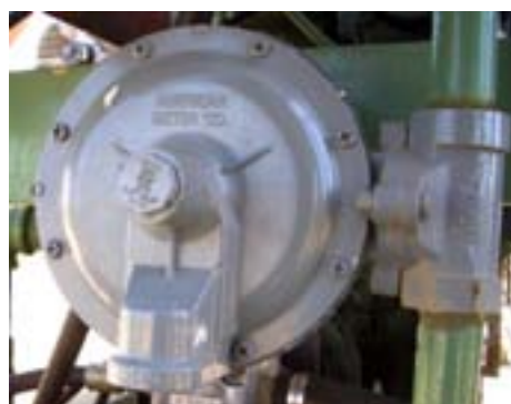
Figure 21. Second-stage pressure regulator used in vapor service.
