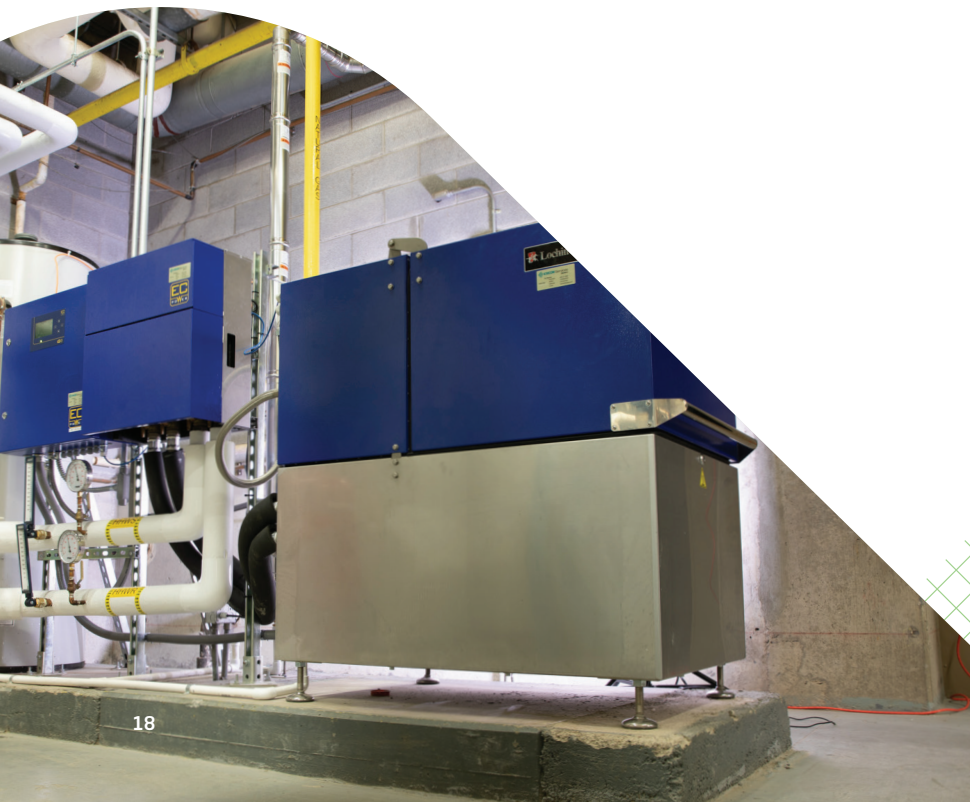
A Lochivar XRG1 25 micro-CHP system installed at Finger Lakes Community College in Canandaigua, New York, produces 24 kW of power and 163,000 Btus of heat.
