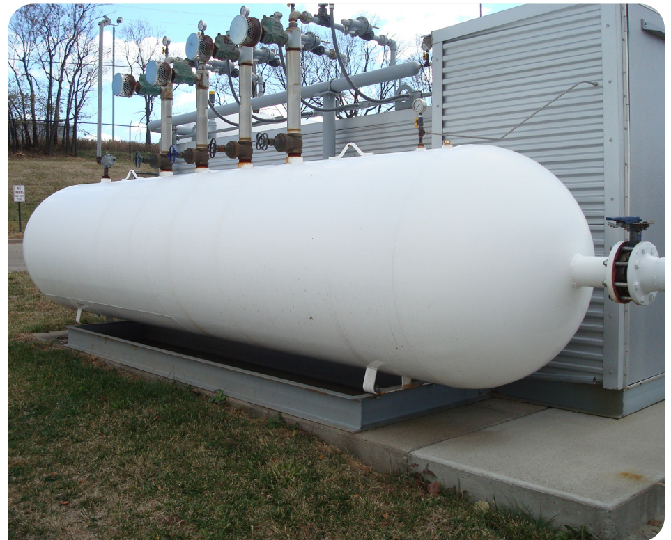
A standby propane system consisting of a propane-air mixer and water-bath vaporizer designed by Superior Energy Systems.
