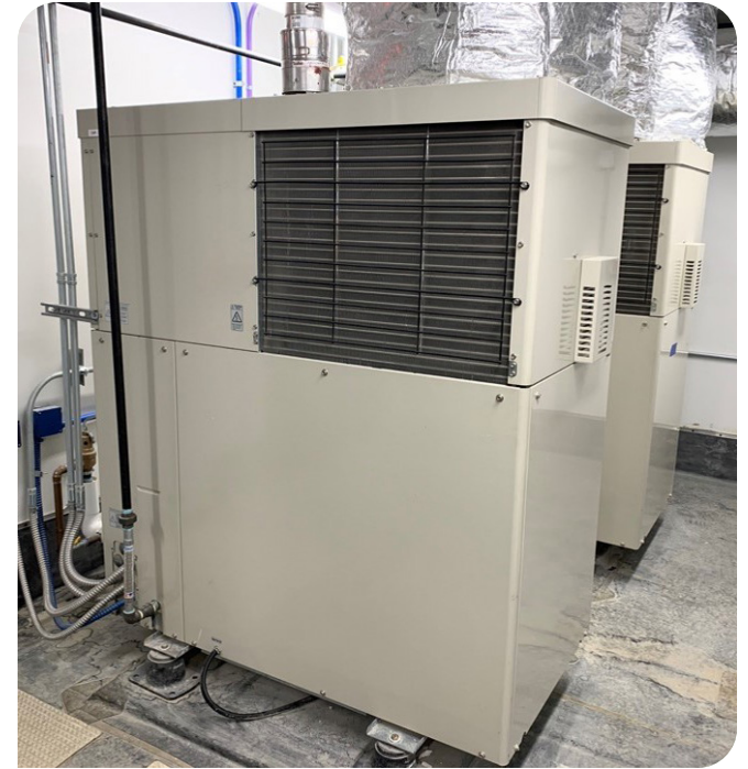
At the Maine Army National Guard’s Northern Maine Readiness Center, two 10-kW micro-CHP units provide domestic hot water and primary heating for the building’s radiant slabs.
