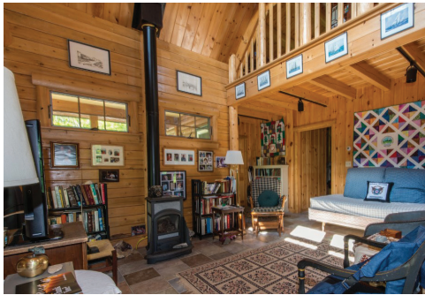
The home's domestic hot water and in-floor radiant heat are provided by a propane boiler, while a propane soapstone heater can be manually operated between seasons.
