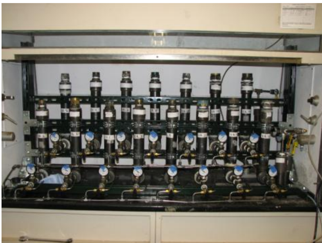
Figure 22. PRV Conditioning Stand
